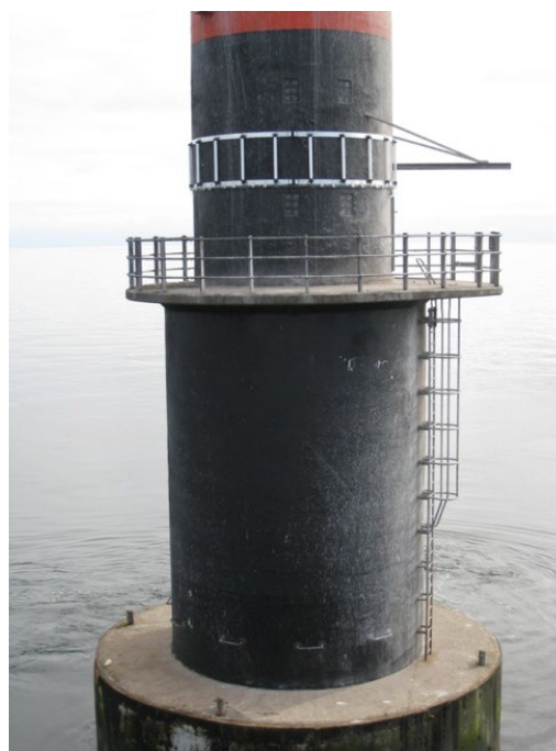
Figure 2 Almgrund Lighthouse, Sweden, equipped with LED pipes
