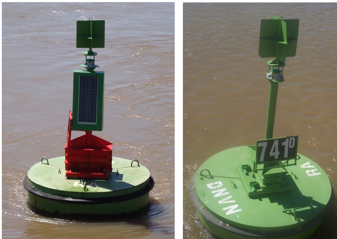
Figure 7 Example buoys with robust steel battery boxes and solar panel.
