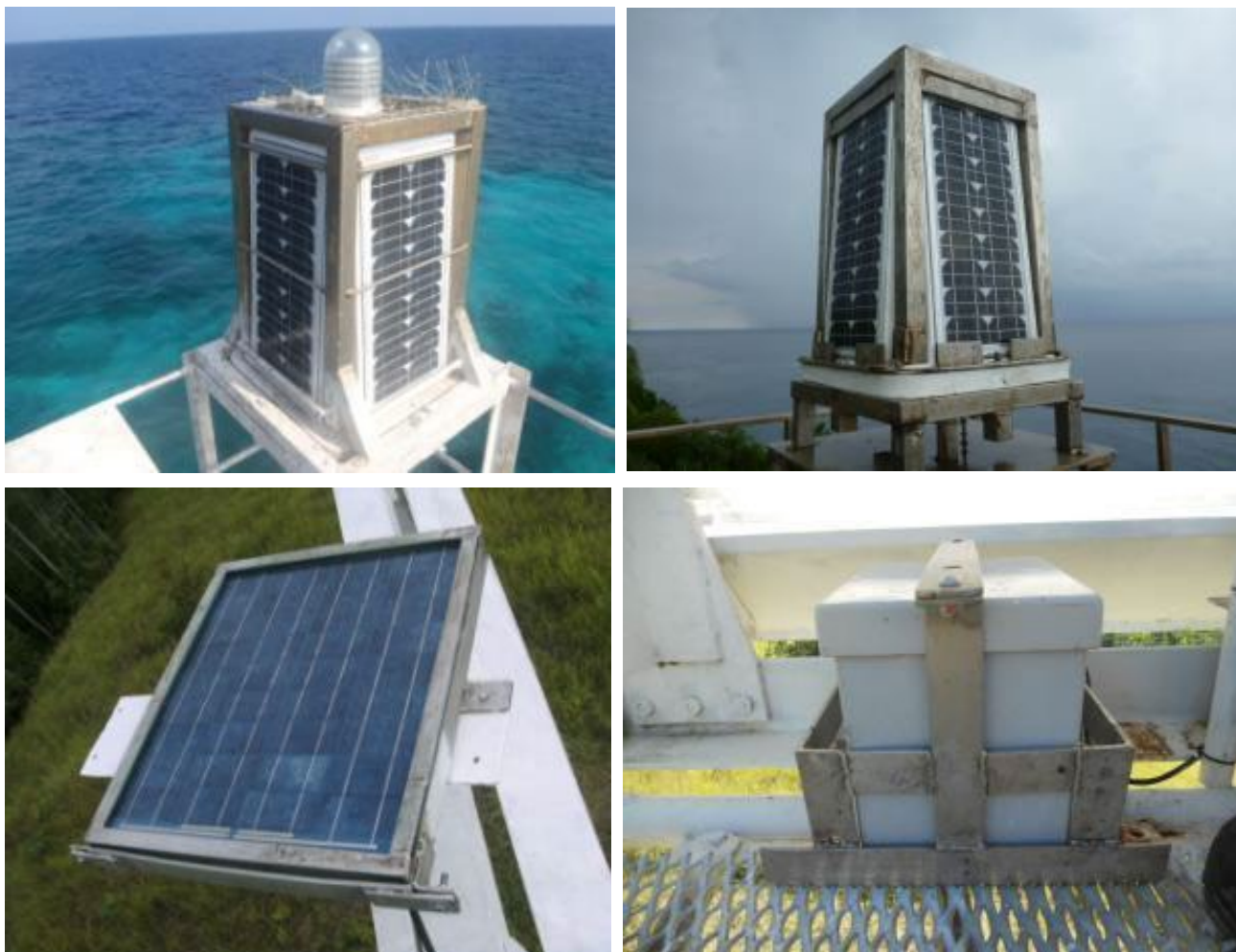
Figure 11 Examples of engineered methods of theft deterrents, including fabricated stainless steel security frames for batteries, solar panels and lanterns.
