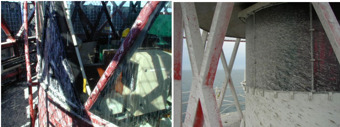
Figure 4 Examples of bird fouling accumulating on lighthouse glazing (Source: Trinity House and Danish Maritime Authority)
