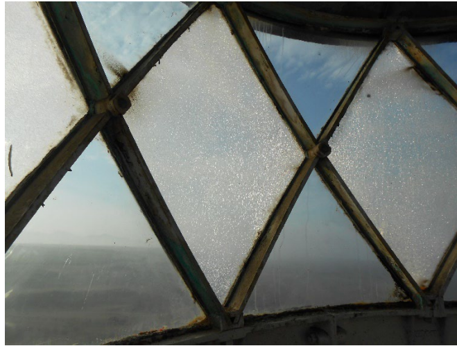
Figure 5 Example of different degrees of degradation of glazing panels made from plastic (diamond) and glass (triangular). Source: MSM
